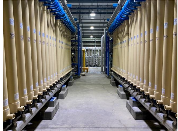
Figure 2. MF Racks at Yucaipa
