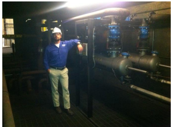
Superior's Capital Improvement Project Manager with two B6-180 model filters.
