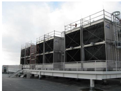
CJIS cooling towers
